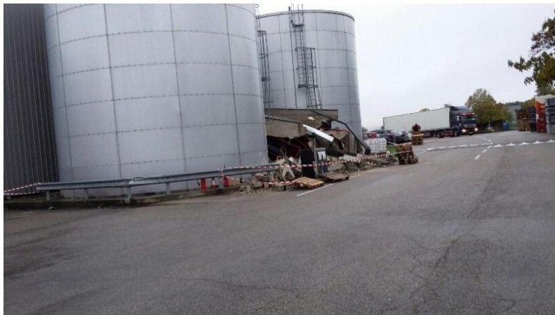
The pump house destroyed in the October 2016 explosion.
